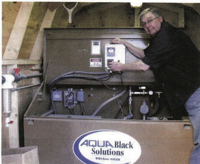
EJB's plant manager Jim Marks (above) says in addition to solving its over-amping problem, the Maxam foaming system the company installed has allowed them to increase RAP percentages from an average of 15% to 23%.
