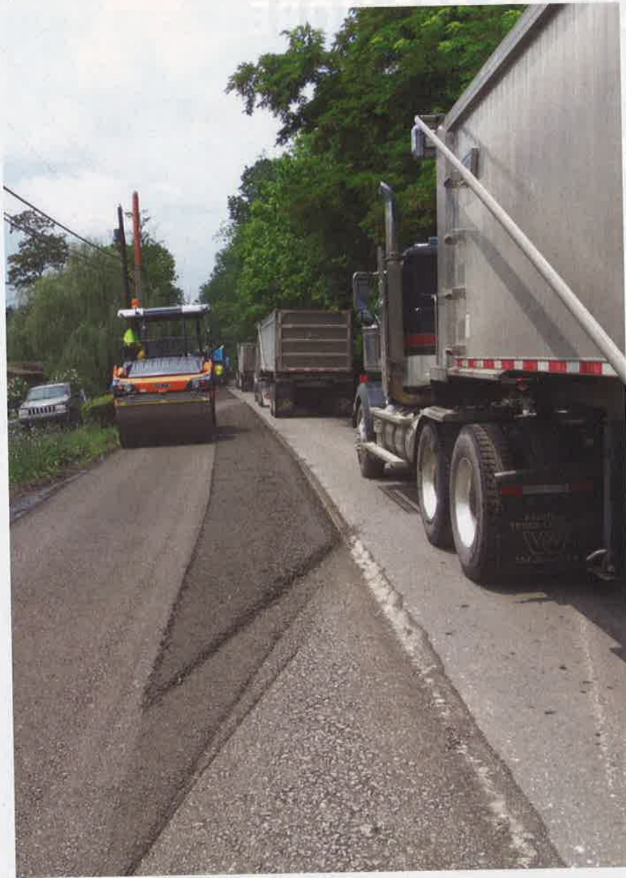
CIR base being compacted, heavy truck traffic hauling coal along Fort Martin Road.
