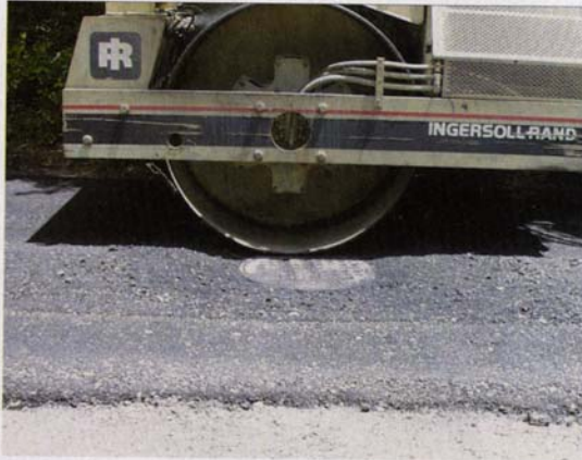
A steel-drum roller compacts the cold-recycled asphalt around a manhole cover. Crews use compact equipment to mill around such structures before the recycling train makes its pass.
