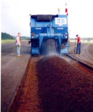
Cold in-place recycling followed the laying and rolling of the RAP. Here, the CIR machine windrows processed asphalt and RAP for placement by a trailing paver. To the left of the windrowed course is placed and compacted recycled material; to the right is the old pavement topped by 3 inches of RAP. To help maintain the cross slope, Breneman made all the CIR passes in the same direction, backing the machines the length of the runway after each pass.
