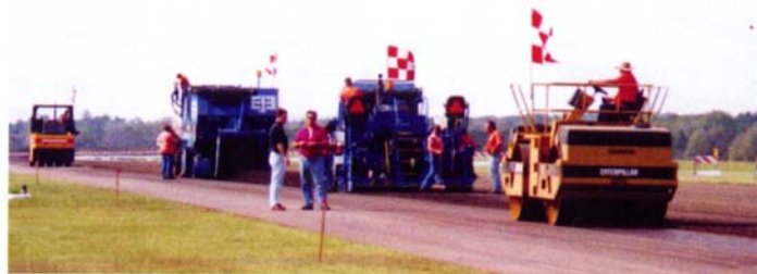
The full recycling train works on the Quincy-Gadsden runway, lead by Breneman's mill, then the Barber Green paver and windrow elevator. A 30-ton Dynapac pneumatic roller and a 12-ton Cat tandem steel-drum vibratory roller work the CIR base from the previous pass. The tandem roller was used for initial compaction — and in static mode for finish compaction. In between, the pneumatic made as many passes as necessary to achieve the target density.
