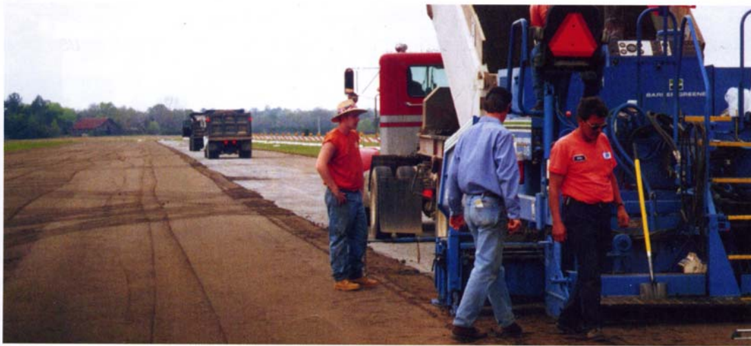
A Breneman crew uses a paver to precisely place imported asphalt millings to a depth of 3 inches over the entire runway. The RAP was then compacted. Grade was checked behind the paver using the string line and a Spectra Physics level. A cross slope of just 1% was allowed. The process took two days.
